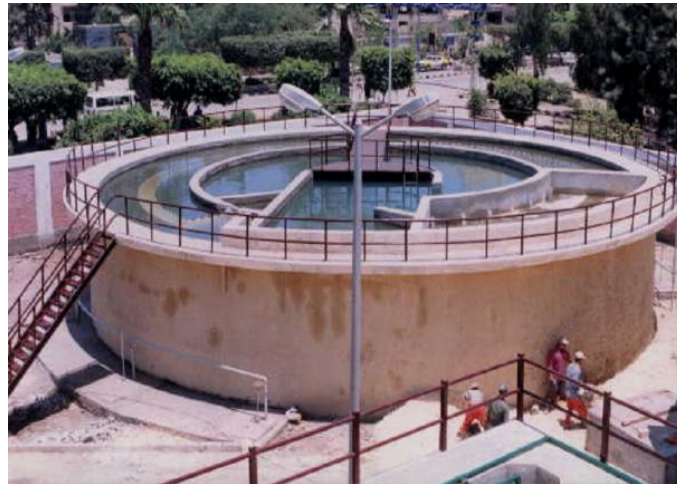
Photo 3 The upgraded circular sedimentation tank.
