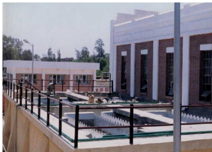
Photo 4 The upgraded rectangular sedimentation tank.
