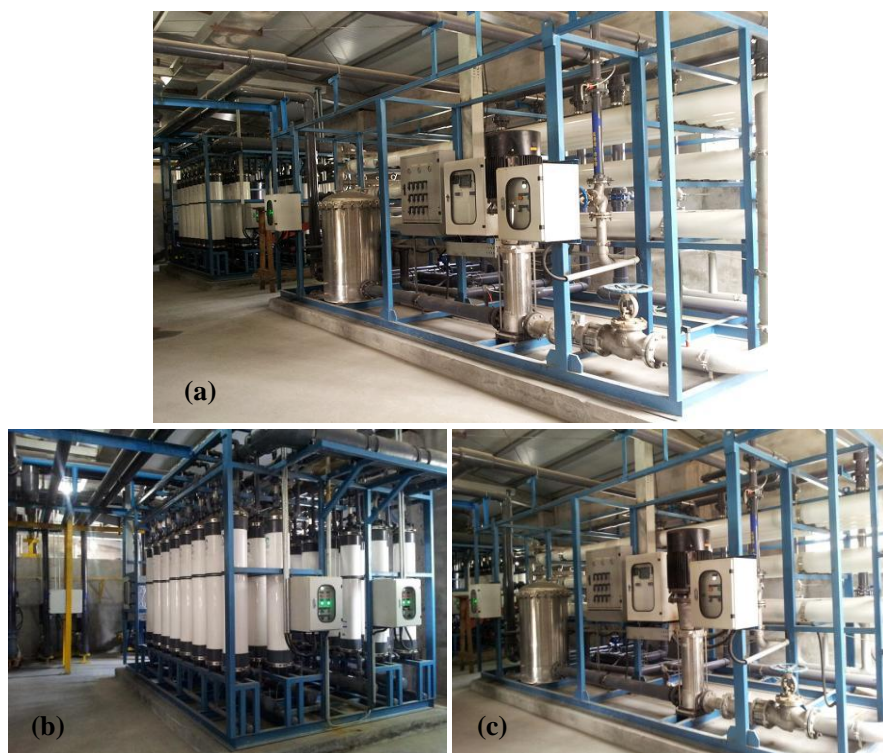
Figure 2 The photographs of the full-scale electroplating wastewater treatment plant: (a) a full view of the integrated UF/RO system (b) UF installation, (c) RO installation
